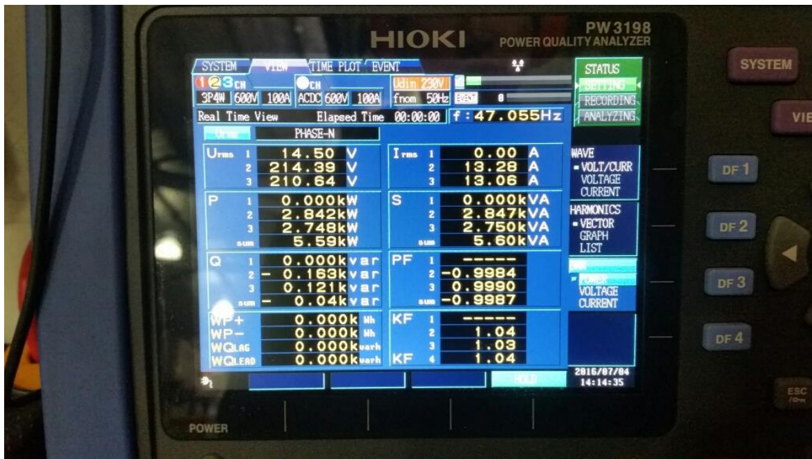
Figure 11 – Power analyser screenshot at 5.59kW
